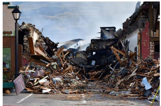
Fire damage in Gardiner, MT. (Graeden Roesler photo for Billings Gazette)
