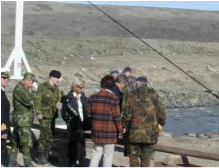
Col Whitehead, Commander Soegaard and Chiefs of Defense visit damaged bridge from recent flood
