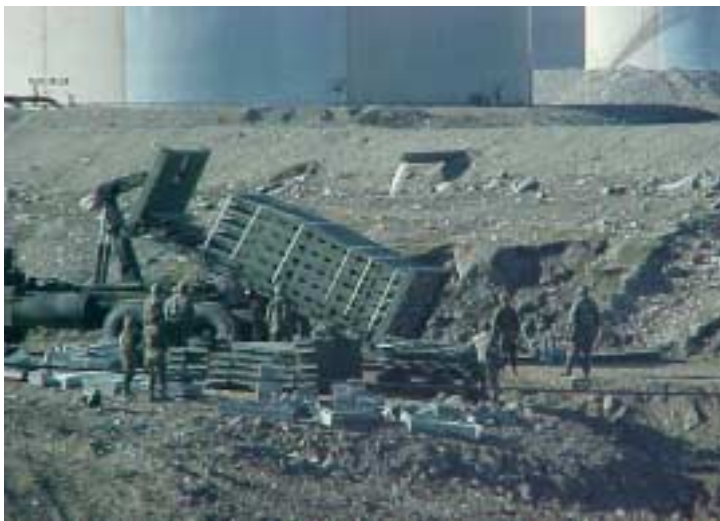
62nd Engineer Battalion, Ft. Hood, Texas building a bridge to north POL
