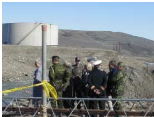
Col Whitehead, Commander Soegaard and Chiefs of Defense visit damaged bridge from recent flood
