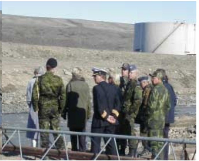
Col Whitehead, Commander Soegaard and Chiefs of Defense visit damaged bridge from recent flood
