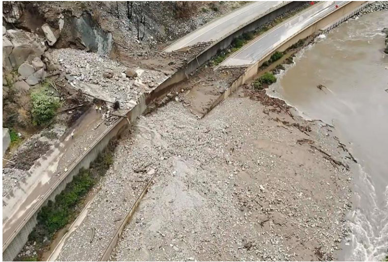
Flood waters caused a landslide across I-70, and reconfigured the Colorado River east of Glenwood Springs
